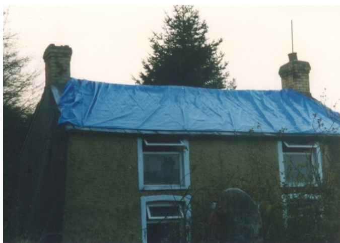
Troedrhwy Llanc cottage, before repairs
